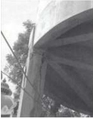
Fig -5: Elevated Water Tank of Gujarat, Located in India after the Occurrence of Bhuj Earthquake in 2001 [3]
