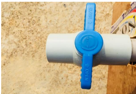
Fig 7: Gate valve or slurry out let valve
