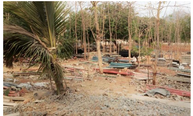
Fig - 5: Materials stored in unorganised manner - 1
