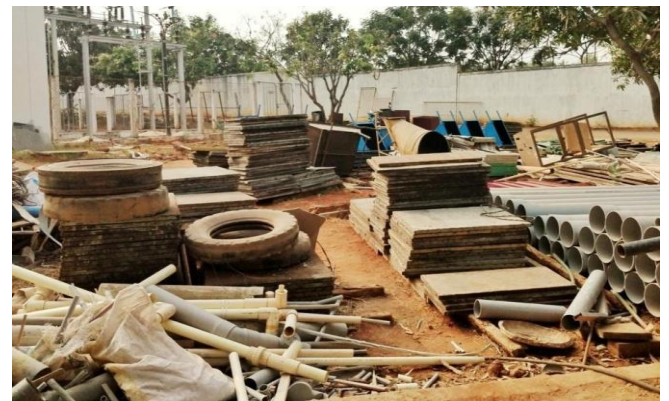
Fig - 6: Materials stored in unorganised manner - 2
