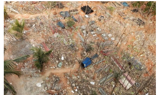
Fig - 7: Materials stored in unorganised manner - 3
