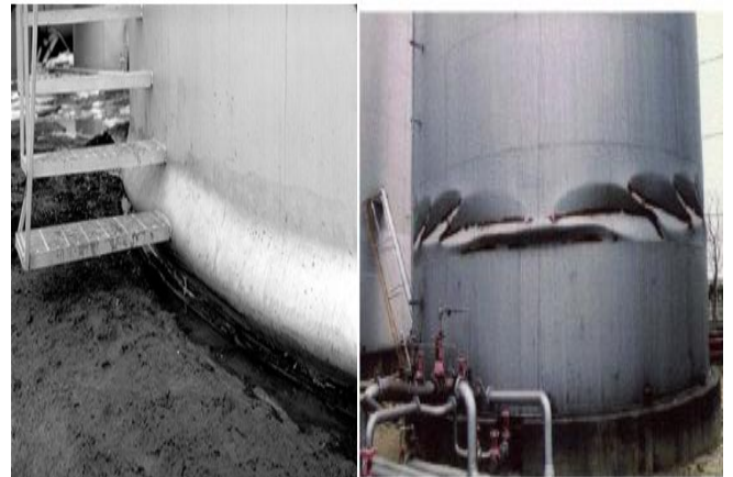
Fig -3: Shell Buckling
