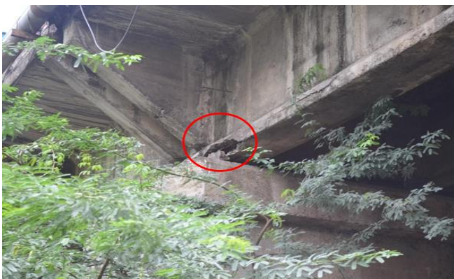
Image-5: damage to the structure at bearing location
