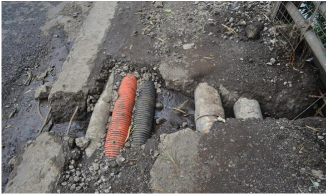
Image-2: service lines in footpath are not covered
