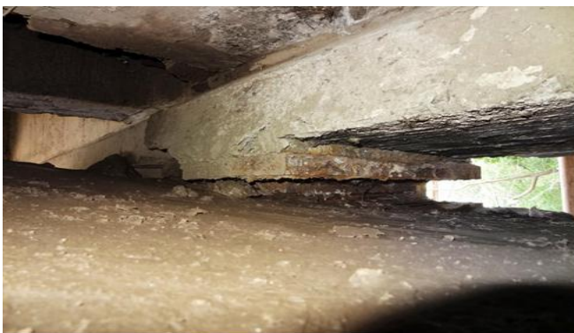
Image-4: Damaged bearing
