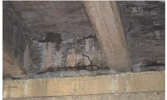
Image-6: Damage in deck slab, steel is open in slab
