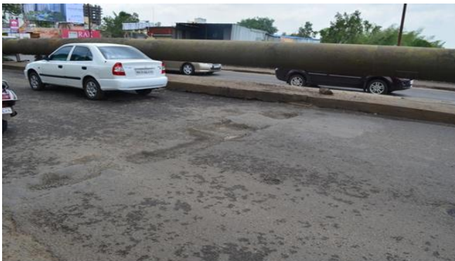
Image-3: Expansion joint are to be damaged
