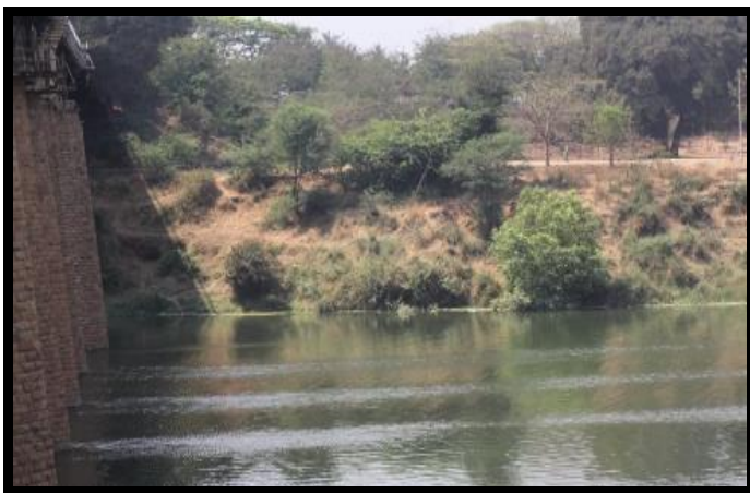
Fig7:- absence of training wall in river bed
