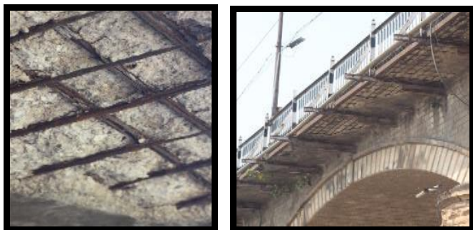
Fig.6:-Spalling of concrete of deck slab
