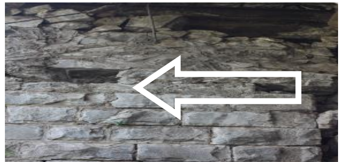
Fig3:- Delamination of stones in abutments
