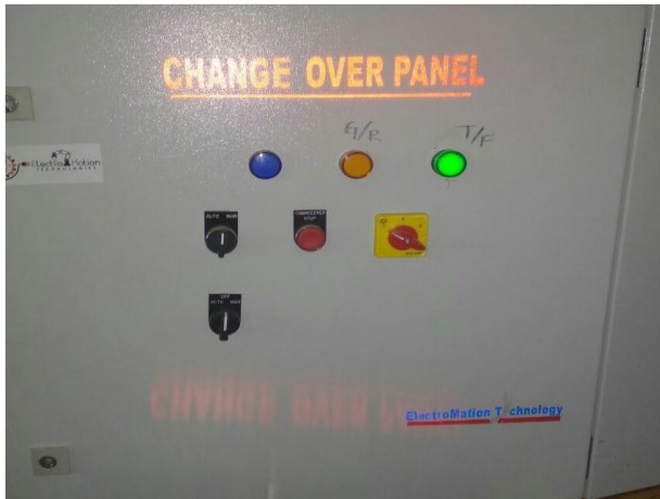
Figure-8: When transformer supply is interrupted, ATS will shift its position from transformer to diesel generator through PLC command and then turn off green light and on orange light in the panel which we can identify which supply is feeding to the load.
