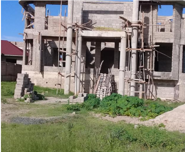
Figure 30: Over-designed Reinforced Concrete Double Columns of a Two Storey Residential House Source: 2018 Field Survey in Mbweni-Dar es Salaam
