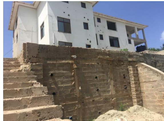
Figure 25: Poor Architectural and Structural Design Considerations on Housing Cost Source: 2018 Field Survey in Dar es Salaam
