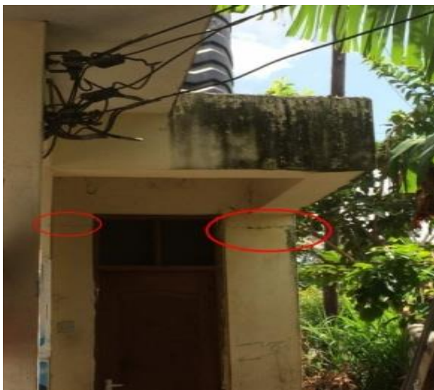
Figure 31: Loading Water Tank without Proper Structural Designs may Results onto Wall Structural failure Source: 2018 Field Survey in Mbweni-Dar es Salaam
