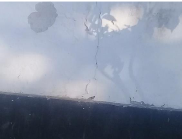
Figure 34: Growth of algae as Result of Poor Green Landscape Architecture Close to External Walls Source: 2018 Field Survey in Mbweni-Dar es Salaam
