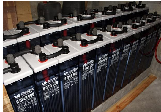
Figure 3. Photovoltaic system array (a) and accumulation system (b)
