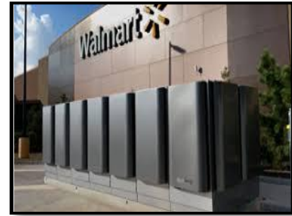
Fig-7: Bloom Energy Servers Installations
