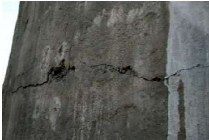
Fig -3: Major Horizontal Cracks
