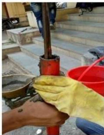
Photo-2: Casing pipe filled with concrete during the fabrication process of buckling restrained brace
