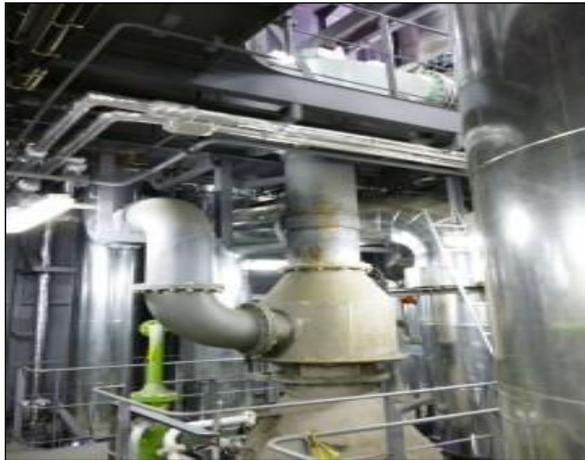
Fig – 6: Deplume reheater unit
