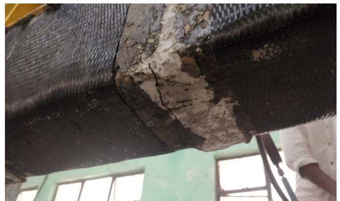
FIG-9: Failure mode of strengthened beam
