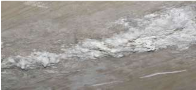
Fig. 7: Spalling of concrete due to sulfate attack
