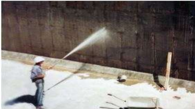
Fig. 23: Surface preparation by water jetting for surface applied coating of crystalline water proofing
