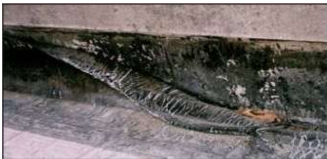
Fig. 12: Damaged sheet membrane
