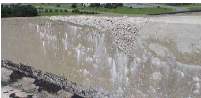
Fig. 4 : Freeze Thaw damage to concrete
