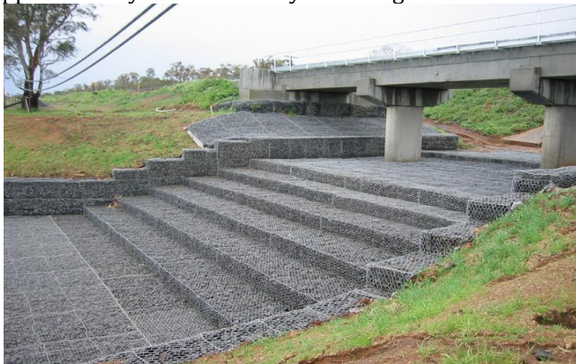
Fig -4: An Apron of Gabion, protecting the stream bed from being scoured.
