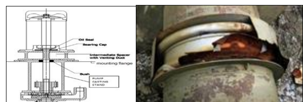
Fig -1: Existing System and its Failure.
