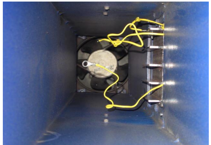
Fig -10: Magnified view of the five-fin sample installed inside the air duct
