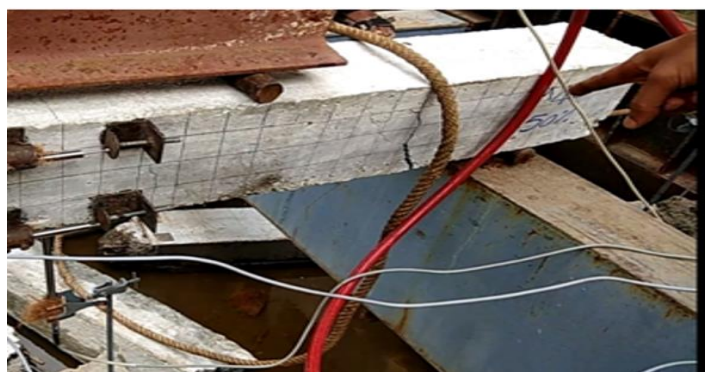
Fig 4.11. Crack profile for RC beam with 50% lapping
