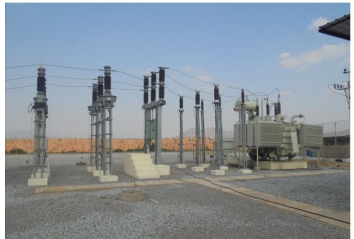
Fig-6: 66KV switch yard
