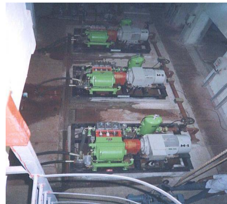
Figure1: High pressure pump unit
