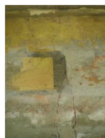
Spalling of Brick of 7-Layer Red Brick Prism
