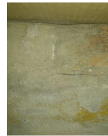
Bond Failure of 7-Layer Red Brick Prism
