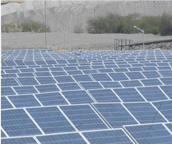
Figure 7 - Solar park for harvesting solar energy at large scale [16]
