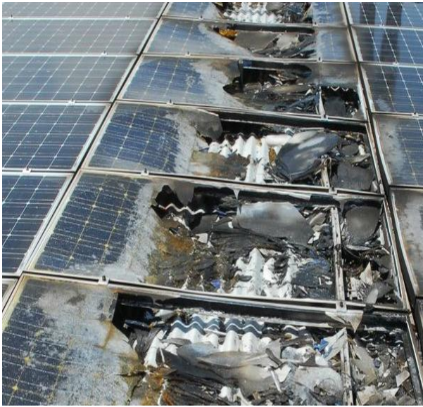
Fig 1.1 (b) fault occurred in 1 MW PV power plant in Mount Holly, North Carolina, in 2011
