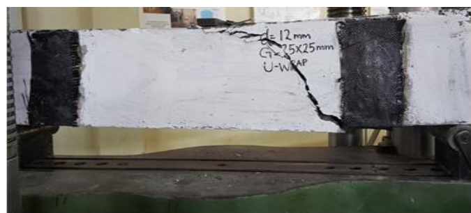
Fig -10: Shear failure in UBD12G25
