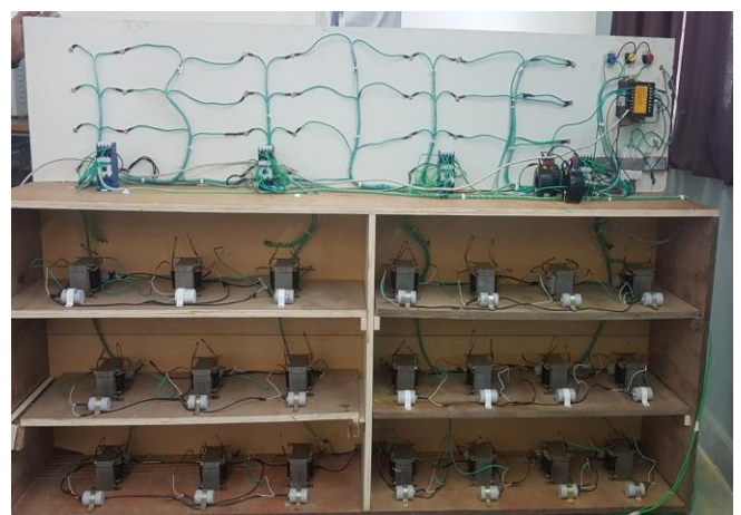
Fig 4:- Photograph of Back View of Pane
