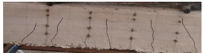
Fig-11 Crack pattern for beam having 60mm middle layer thickness (T4)
