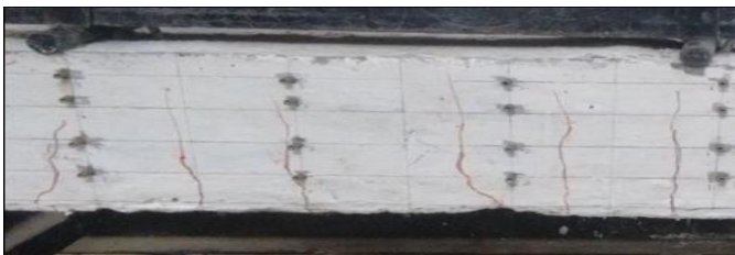
Fig-7 : Crack pattern for Control beam (CB)
