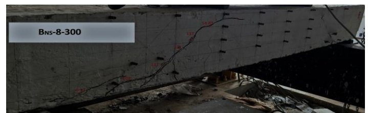
Fig -5: Crack pattern of BNS-8-300
