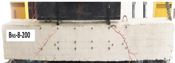
Fig -8: Crack pattern of BNS-8-200
