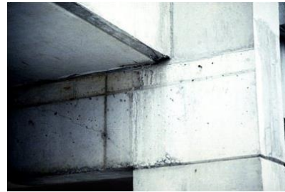
(a) A diagonal shear crack occurring in a reinforced concrete beam near its connection to a column
