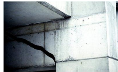
(b) A manipulated version where the portion of the beam below the crack has been moved down to emphasize the mode of failure
