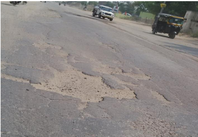
Fig.-3: Formation of ruts, cracks and pot holes nearby Gangwa Village, Hisar.
