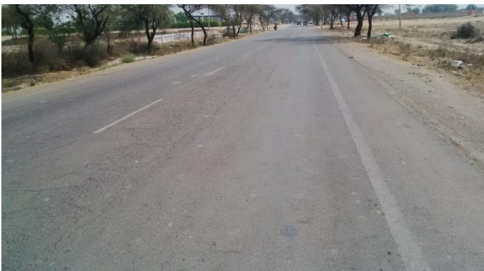
Fig.-4: Poor pavement markings and maintenance nearby Chaudhriwas Village, Hisar
