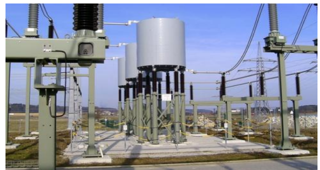
Fig.2:- Current Limiting Reactor (CLR)
