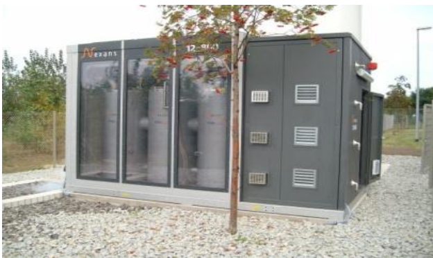
Fig.3:-Super conducting fault current limiter (SCFCL)
