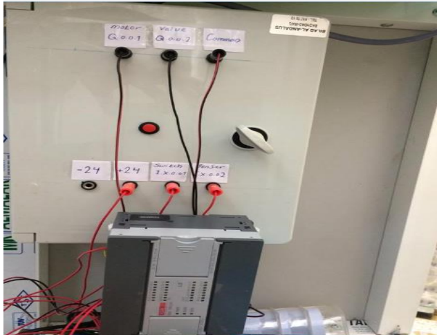
Fig-13: The Automatic control Panel.
