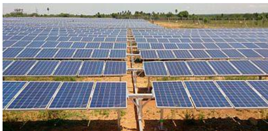
Chart-12 Solar power plant
