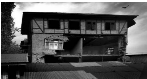
Fig -9: House in Kashmir damaged in 2005 earthquake showing how unreinforced masonry collapsed, leaving the top story of Dhajji Deewari in place. [4]
