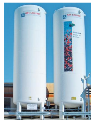
Fig:1.1 Pressure Vessel for Storage(Nitrogen)
