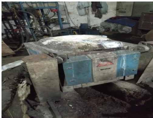
Fig -1: Electric Resistance furnace
