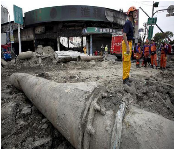
Figure.12. Corrosion in pipelines
