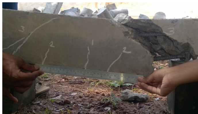
Fig -6: Cracking pattern of Control beam with normal steel
