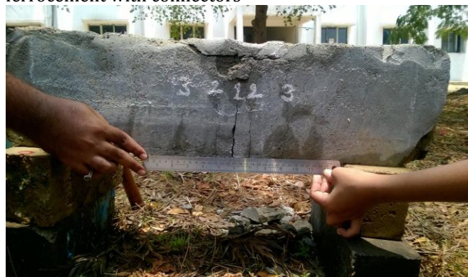
Fig -10: Cracking pattern of jacketed beam by 3 layer mesh at orientation of 45 degree reinforced ferrocement with connectors
