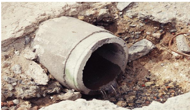
Fig -2: Circular Gutter Channel
