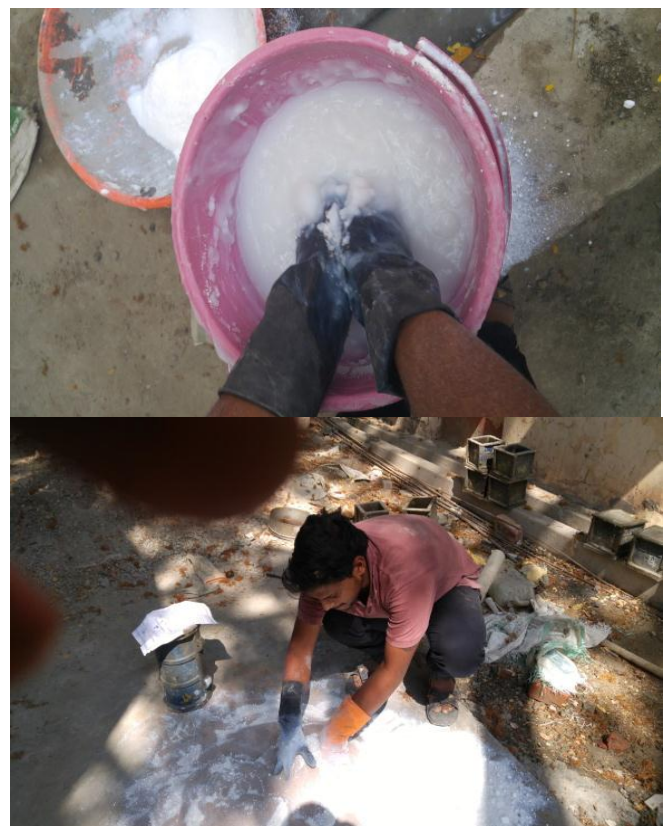
Fig 1: Types of mixing Nano-silica with super plasticizers water solution and with fine aggregates
