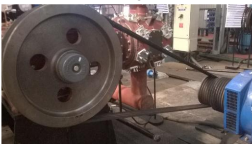
Fig 1.1 Motor compressor setup
