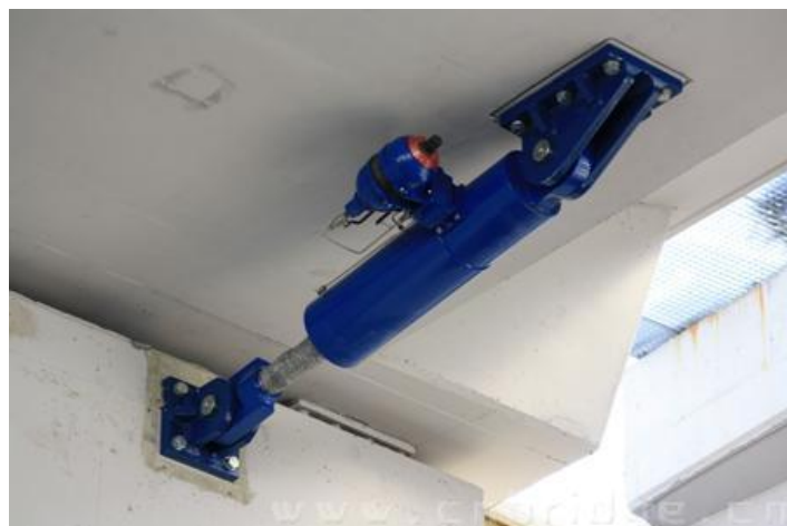
Fig-3: A fluid viscous damper installed on a bridge
