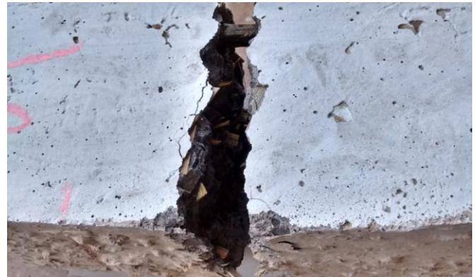
Fig.: 10 failure of the beam in flexure
