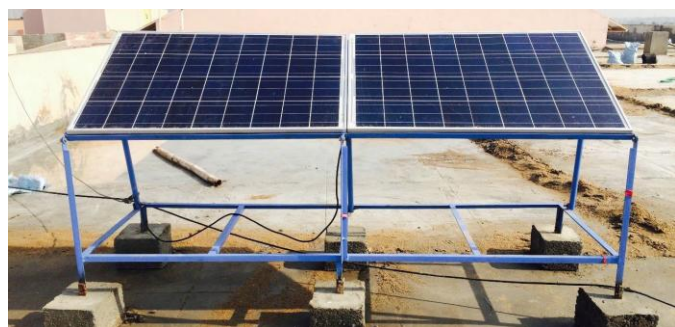
Fig.1 Solar panel mounted on the frame
