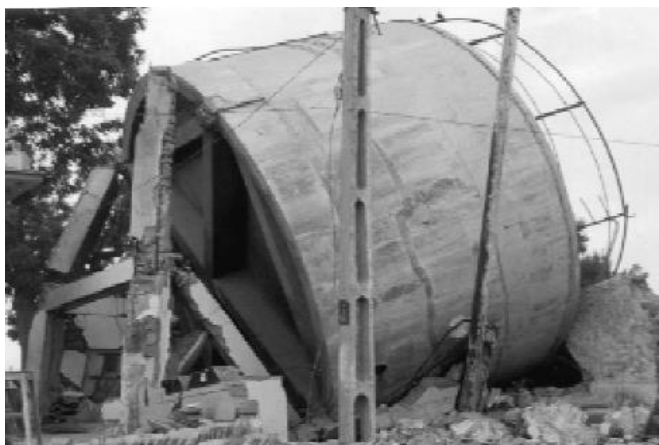
Figure 2 Collapsed water tank in Bhachau (Source: Rai, 2003)
