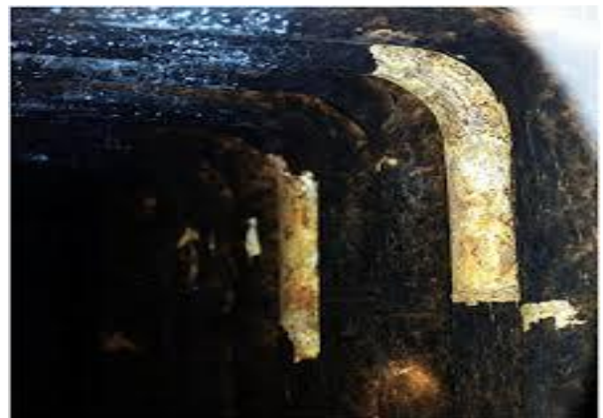
Fig -2: Oil Ash corrosion on water Panel Bends
