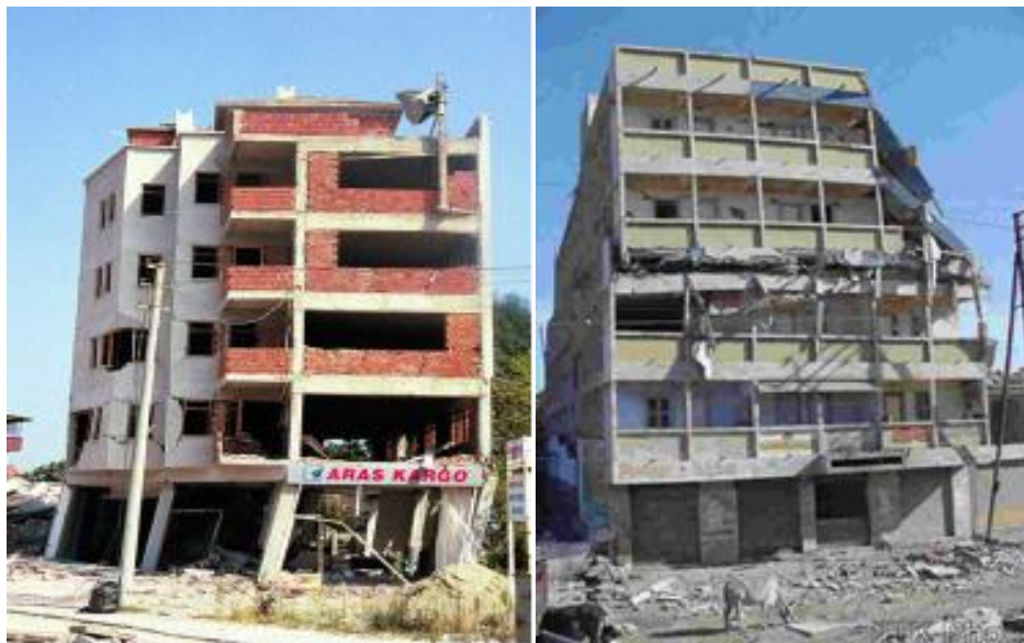
Fig 3(a) Ground soft storey failure, Fig 3(b) Intermediate soft storey failure
