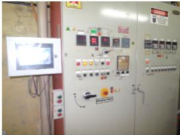
Fig- 9: Old control panel cabinet is used for our work
