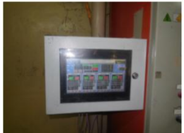
Fig- 8: Installed HMI
