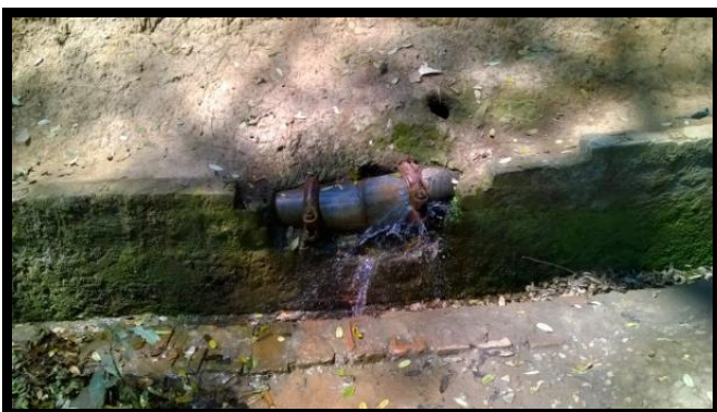
Fig -1: Water getting wasted at a fault location in pipe network of Guwahati City
