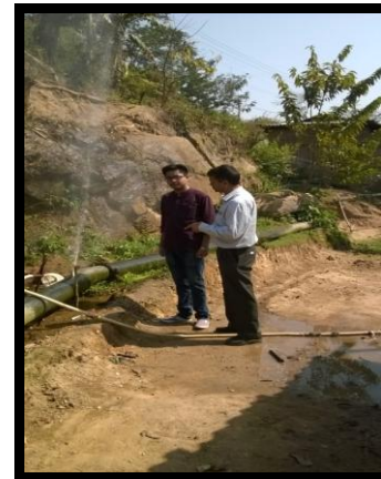
Fig -2: Water splashed through conduit fault
