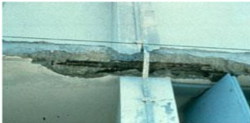
Fig.4: Macrograph of exposed building façade due to carbonation
